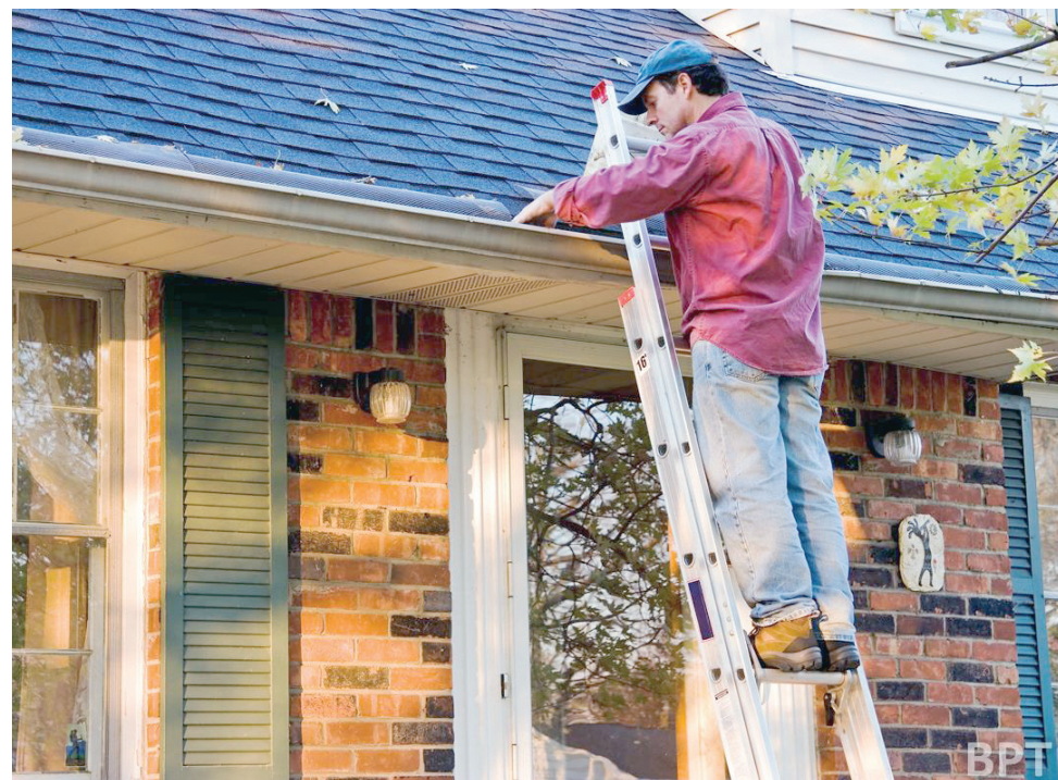
Clear the gutters to prevent a future home disaster.
