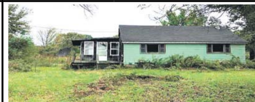
252: 163 Waite Road, AMSTERDAM: Handyman special on a one acre lot with detached 2-car garage. Two bedrooms, one full bath. Property is sold as is. Cash only. Condition of septic is unknown, the cap has fallen in. Caution tape is around the septic, please use caution. A hold harmless agreement must be signed before entering the house due to the enclosed has detached from the house. Asking $25,000
