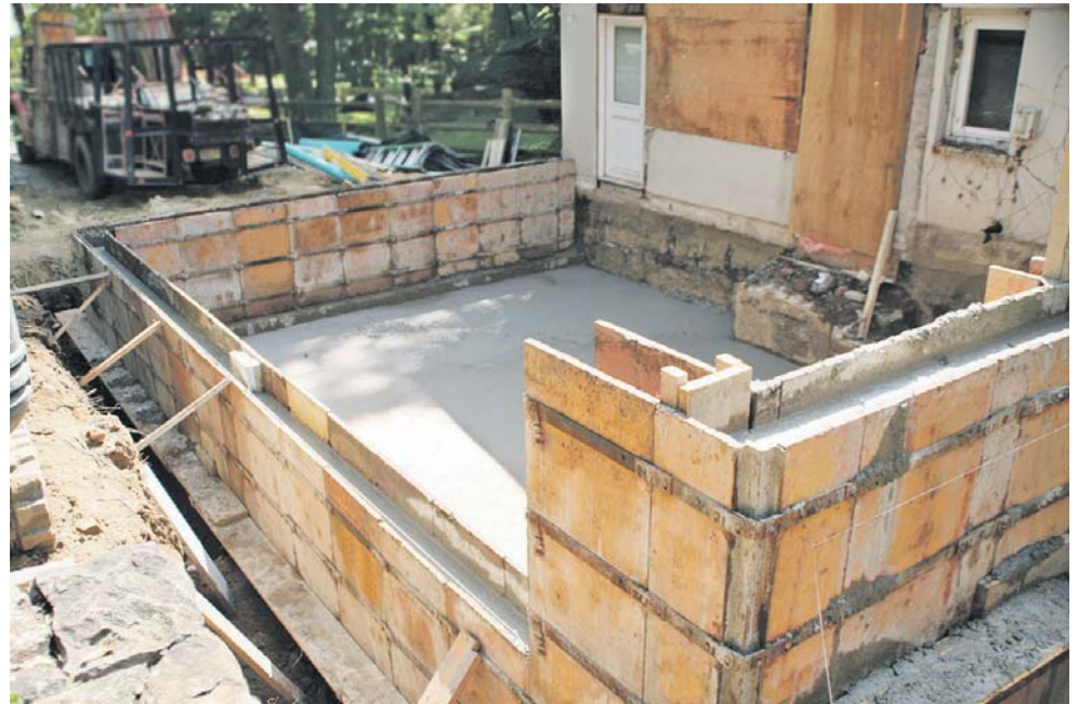
If not properly addressed, ground water can affect an existing foundation and the ability to build successfully.
